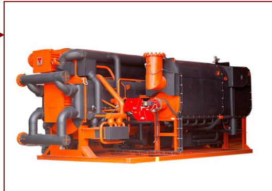
2 x 1300 ton Exhaust gas Fired Chillers with back up firing
